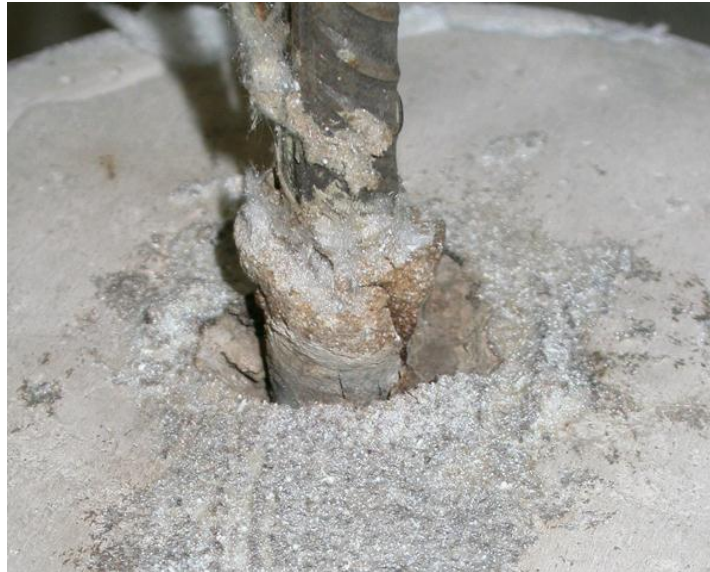
Figure 8: Bond failure after fire exposure
