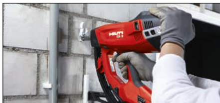
Conduits and light-duty pipes
